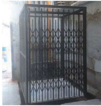
(C-2) COMMERCIAL GOODS LIFT
