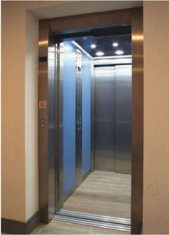
(B-1) PASSENGER ELEVATOR
